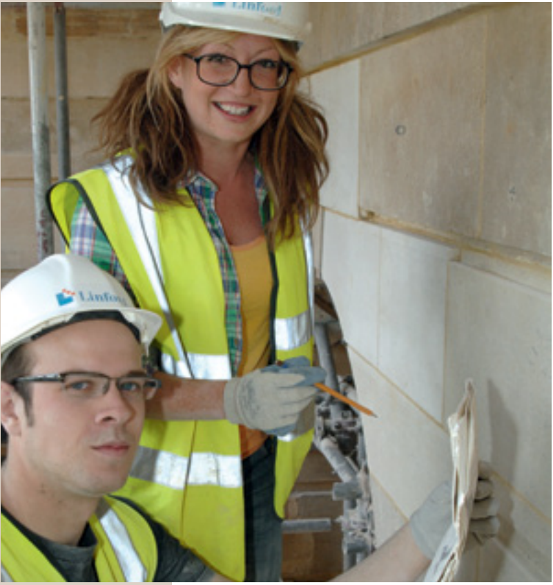
David Pickering and Hannah Baars working on the East Pavilion at Stowe House
